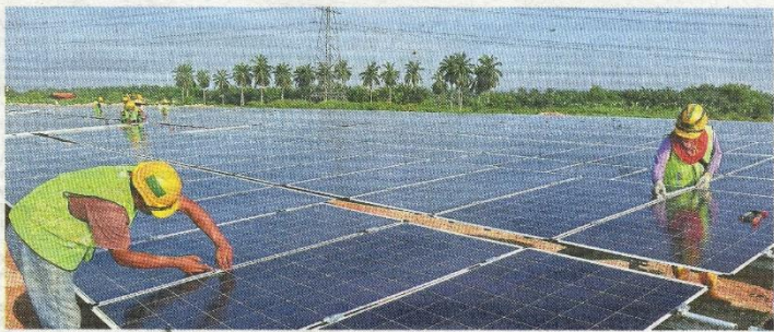
Third round: Contractors installing solar panels at a LSS project site at Kuala Langat. The third round of bidding for LSS power plants attracted 112 companies, with the lowest offering 17.7 sen for 100MW.
